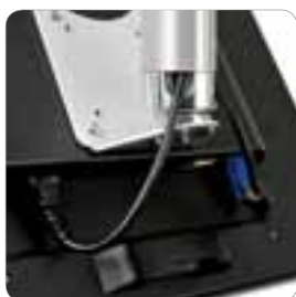
Neatly installed cables
